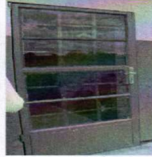
Outer steel door with poor finishes
