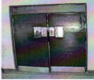
One of the 5 swing wooden double door with poor finishes
