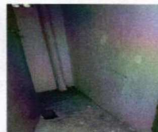
Poor paint finishes and droppings on the floor
