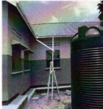
Pipes not fixed
