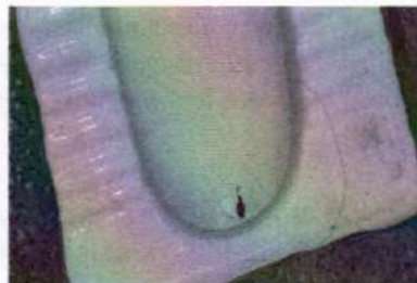
Cracks on squatting pan
