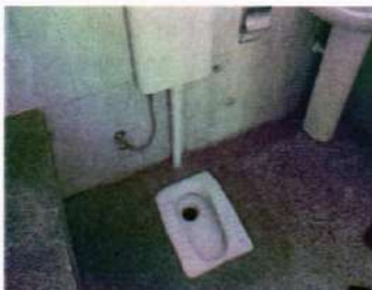
No arm grab rails installed
