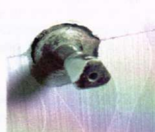
Poor shower tap finishes
