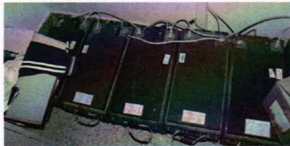
Solar batteries on the floor
