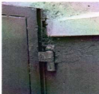
Poor finishes and painting works
