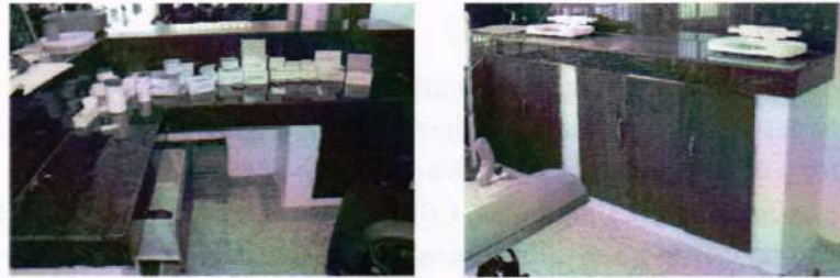
Cabinets with some poor finishes
