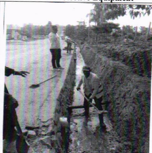
Casual workers desilting a trench without gloves, masks, helmets, overalls
