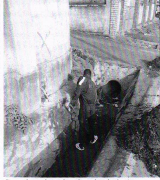
Casual worker cleaning the drainage channel without boots, helmet and gloves
