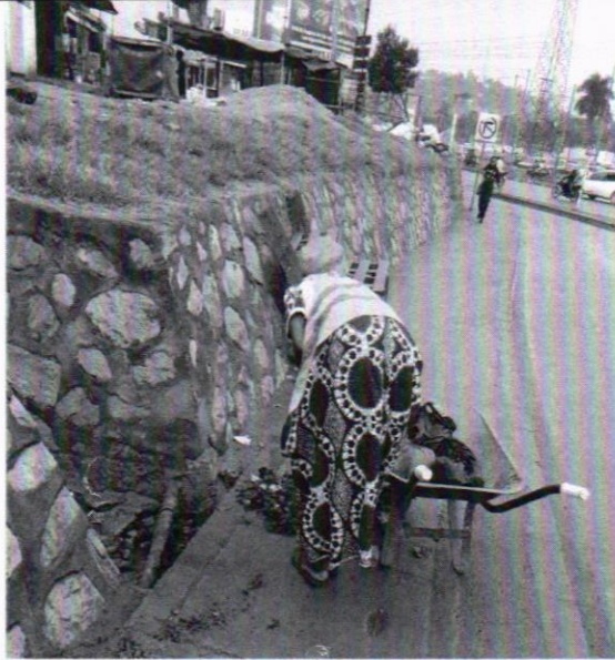
Casual worker cleaning a drain without boots and helmet
