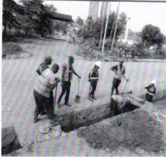
Casual workers desilting a trench without gloves, masks, helmets, overalls
