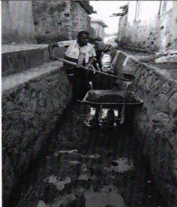
Employee cleaning a trench without mask and gloves
