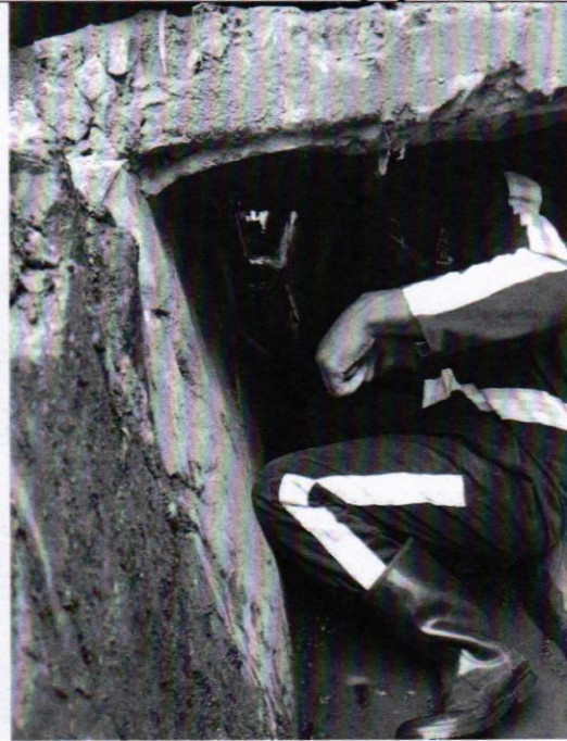
Casual worker unclogging the blocked culvert without gloves
