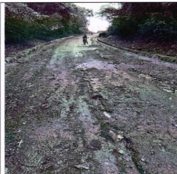
Image 4: sub-standard materials and eroded surface as of 27 th March 2025
