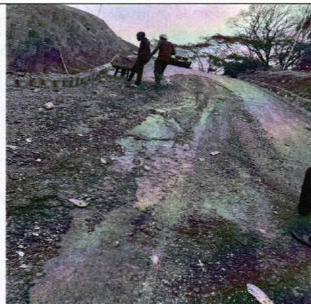
Image 5: Bleeding and rocky surface as of 27 th March 2025
