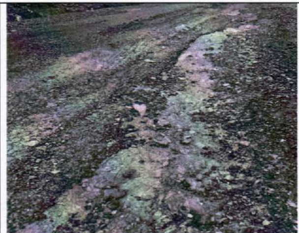
Image 3: Shows a section of a rocky eroded surface
