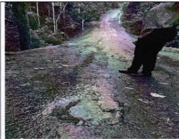
Image 2: shows a section of the road with potholes as of 27 th March 2025
