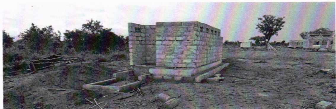
Five Stance VIP Latrine Block for Boys at wall plate level pending roofing
