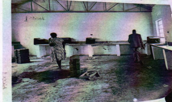
Inside the science laboratory pending some minor installations
