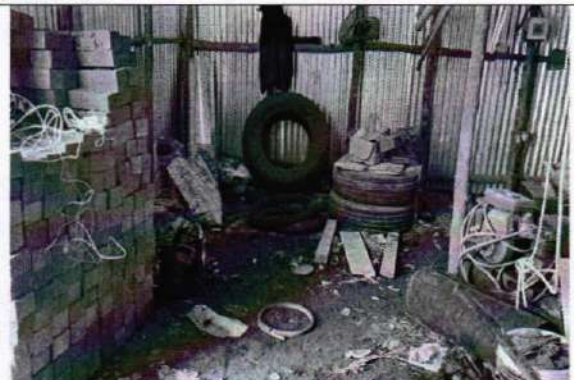
Bricks in store but the store has no doors to protect against theft and harsh weather
