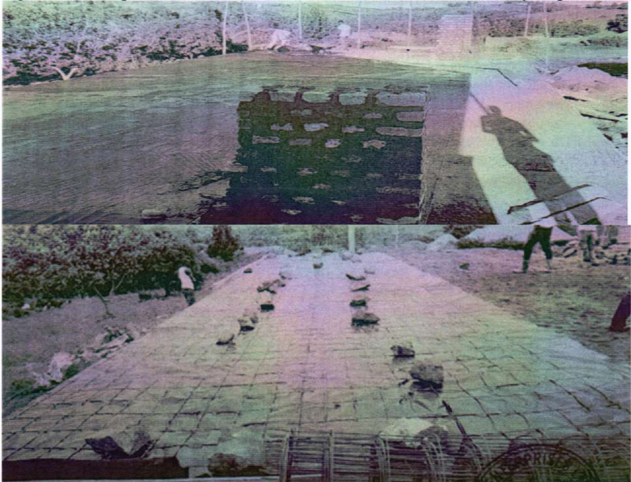
Figure 3: Non-implementation of the Environmental, Social, Health & Safety Requirements
