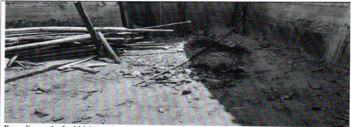
Poor disposal of rubbish on site, with plastic bottles and polythene bags spread all over the site
