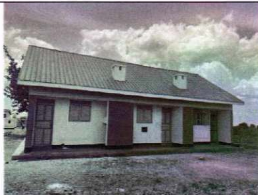
No lightning arrestors, No rumps, no rain water gutters, no water tank, no bathrooms, and no curtain rods
