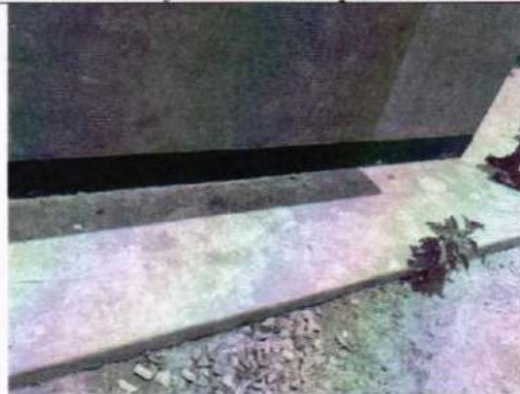
Cracks on splash apron
