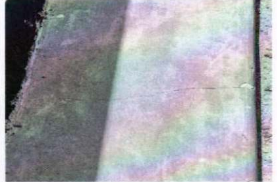
Cracks on splash apron
