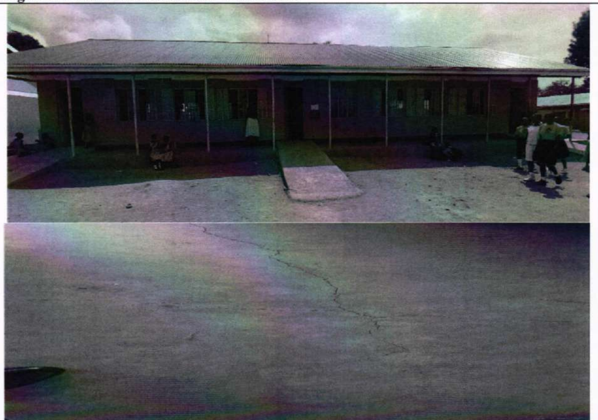
Cracked floor of the store
