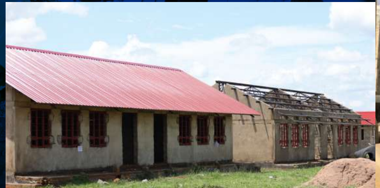
The half-roofed, construction site of Kijunjubwa Seed Secondary School in Masindi district. It seemed less likely that the contractor, CMD Investments Limited would complete the project by the end of June 2024 when their contract expires.
